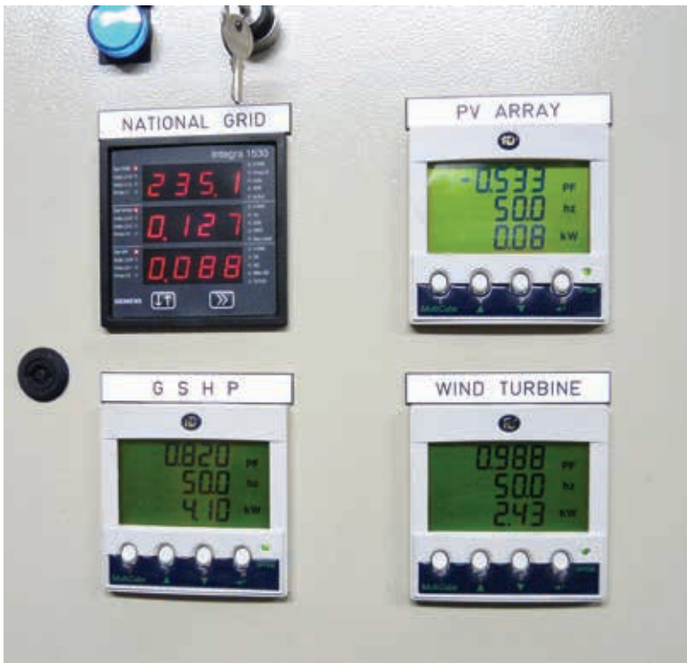
Figure 3: The data panel in the Eco Centre in Cockermouth School, West Cumbria. In 2007, Cockermouth School opened up a unique state-of-the-art Eco Centre, designed for use by students, staff and the wider community. It is engaging over 1,400 students and 200 staff in the energy saving challenge and starting to invest in energy-saving measures and renewable energy. Photo: Ashden Awards.
